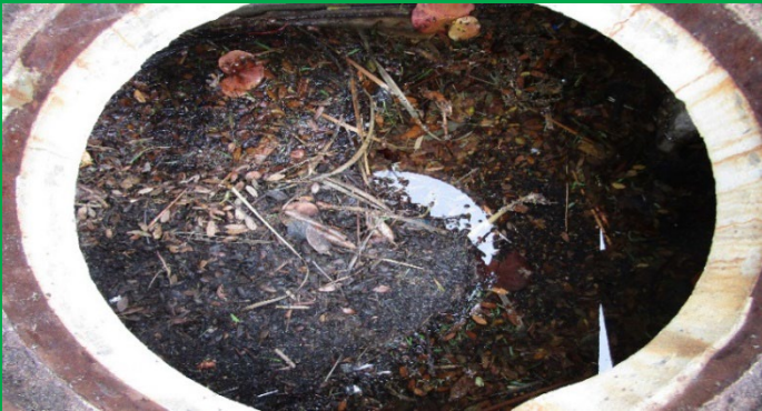
What we find before cleaning stormwater drains
